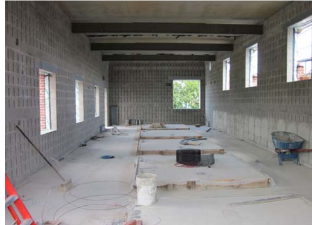
Interior of the New Aeration Blower Building
